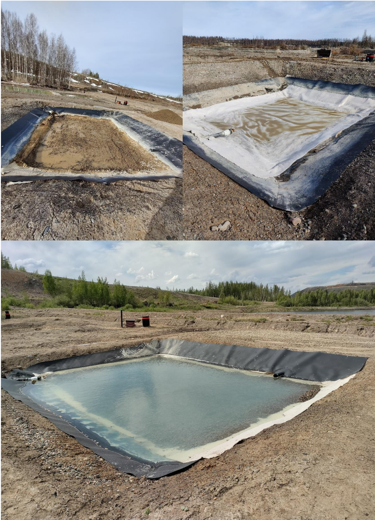
Figure 13. Used old mat after removing of top gravel on the left and new mat on the right, and pilot running in picture on under (Feasib 10.5.2022 and 30.5.2022).
